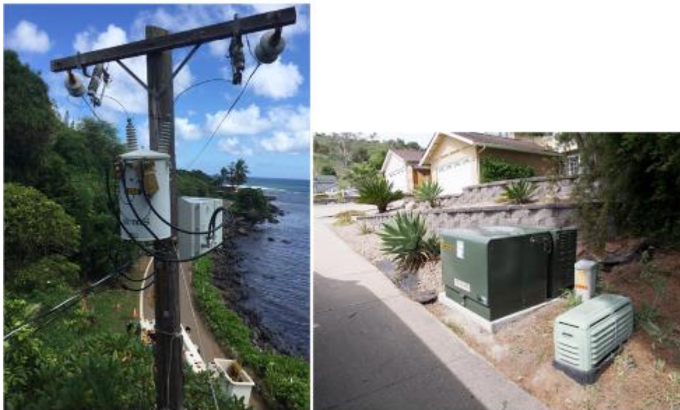
Figure 2. LV Substation implementations for (a) an overhead system and (b) underground plant, featuring coupled integration with a distribution transformer for siting on a standard pad in a residential area. Adding a power electronics-based regulator with integrated sensing, computing, communications and control software brings grid modernization to legacy distribution transformers.
